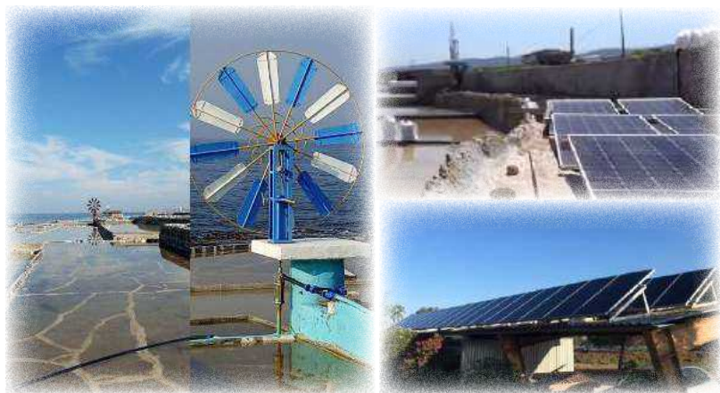
Figure 17. Traditional windmill restored (left), now running with a solar energy-powered pump; and solar panels being installed in the salina (top, right), Sleiman Salinas (Anfeh, Lebanon; MedArtSal project actions). Installation of solar panels (36 in total) on the roof of the car park in Salinas de Chiclana, Spain (below, right). ©MedArtSal project (above) and Salinas de Chiclana (below)
