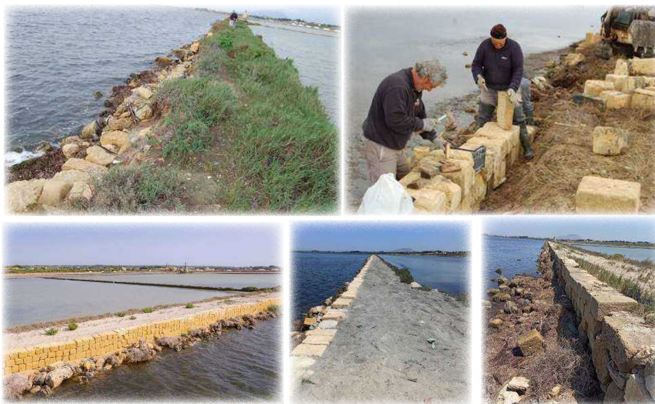
Figure 154. The salt pan's external wall before the intervention (top left); workers at work during the embankment renovation (top right); the embankment after the recovery (middle); details of the embankment (bottom). ©Salina Ettore e Infersa
