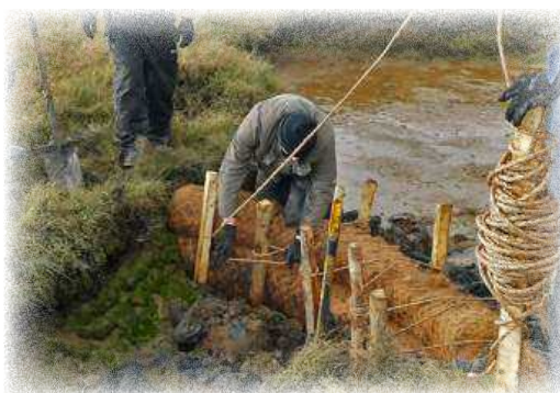
Figure 20. Installing "salt marsh sausages" of coconut coir to try to stabilise degrading coastal habitat. Image courtesy of Essex Wildlife Trust
