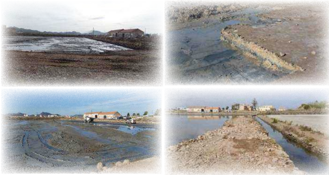
Figure 147. One of the salt ponds (crystalliser) before the intervention (top left), during the works (top right) and once cleaned (below left). The perimeter of the entire crystalliser has been rebuilt (detail of the wall, below right). ©ANSE
