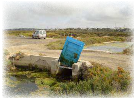
Figure 4. One of the gates controlling the flow of water in Salina La Esperanza (Cádiz, Spain). ©Yana Korneeva Abdulaeva
