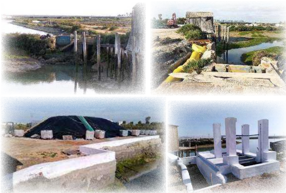
Figure 142. Wall and sluice gate prior to the intervention (above) and after the reconstruction (below). ©Salina San Vicente (above) and H.Clavero (below)
