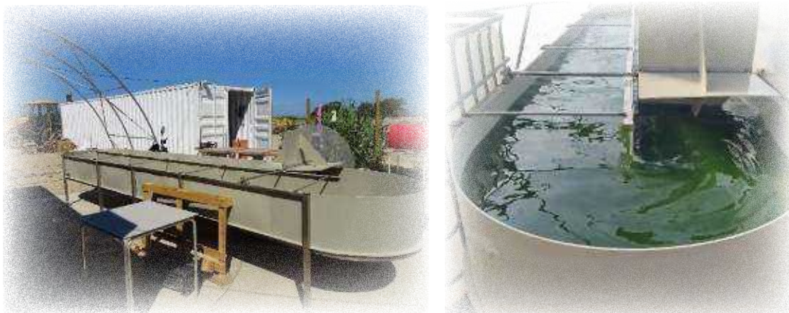
Figure 148. Microalgae cultivation plant during installation (left) and after operation (the reactor with the microalgae; right) in the salina Preciosa and Roqueta, Cádiz, Spain. ©H.Clavero (left) and Marambay (right)
