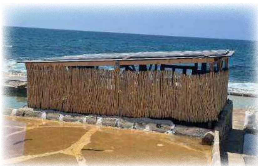
Figure 164. Installation of solar panels on the roof of the hut in the salina. ©Georges Sleiman/Evaura
